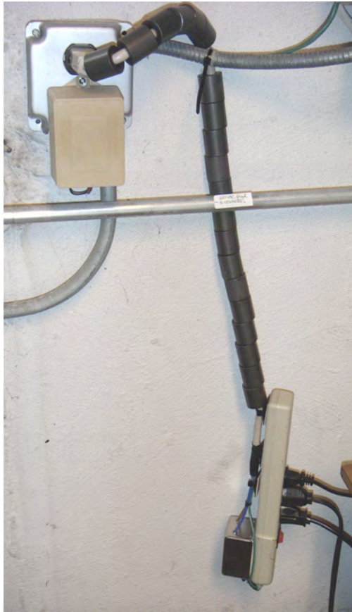
Figure 11: 15-A, 120-VAC, multiple-outlet strip with Corcom two-stage, L-C, difference-mode EMI filter and ferrite-bead common-mode choke added.
